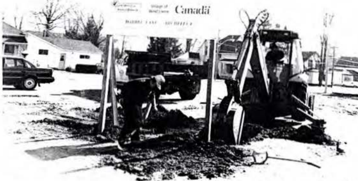
IT'S OFFICIAL: The sign marking the site of the new West Lorne fire hall and municipal complex was erected March 13. Mar-Con Construction donated the use of their backhoe to help dig the hole for the sign, and backhoe operator Dennis Chevalier also donated his time.
