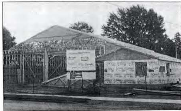
Construction on the new West Lorne fire hall is well underway and it should be completed some time next year. Recently announced cutbacks to projects by the provincial government have not impacted on the project with the Canada-Ontario infrastructure funding left intact. Estimates for the combined fire hall/municipal complex have increased though, currently sitting at approximately $450,000. About $240,000 must be raised locally for the facility.
