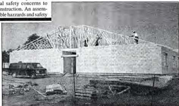
Construction continues on the addition to the St. Mary's/St. Thomas More School.
